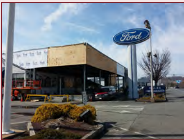
Fred Beans Boyertown Showroom and service department addition and renovations are well underway.
